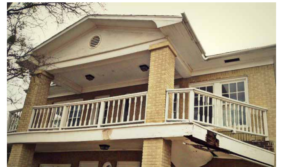
The second-story balcony was sagging and detached from the main structure when the Northerns purchased the property.
