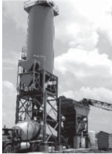
A view of a typical concrete batch plant
